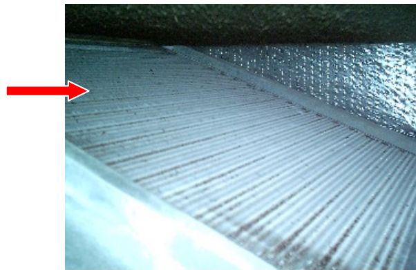
The evaporator coils of the east unit located in the attic area were observed to be minor dirty and should be further evaluated by a HVAC professional to determine if cleaning is needed
