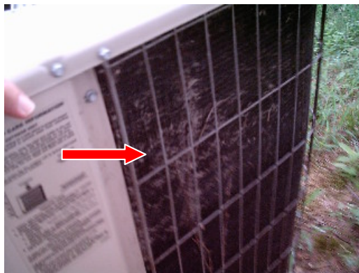
Temperature drop was observed in the far east office. Improvements should be made to the size of the condensing unit to allow coverage of the square footage of the 2 combined office areas
